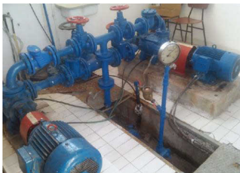
Figure 1. Interior of the PS “Mokra” - previous
