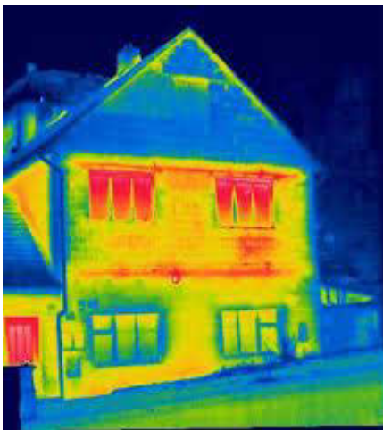
Figure 3. Thermal image showing the temperature of a structure [10].
