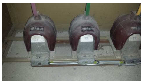
Figure 2. Photo of voltagge measuring transformers during operation – no possibility to read their nameplates
